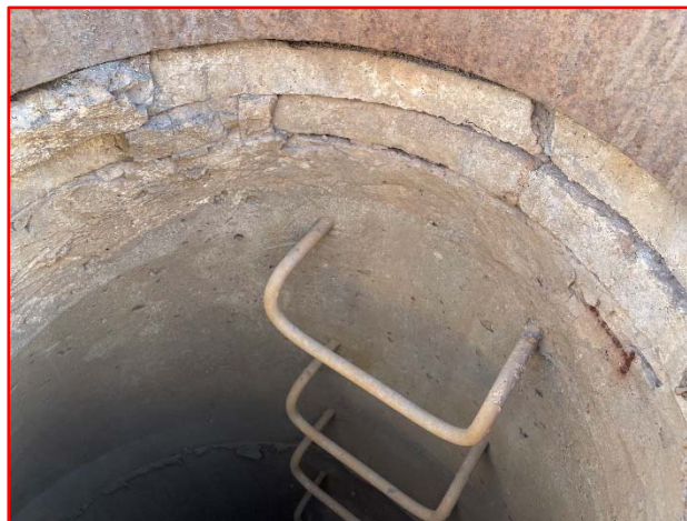
Photo 5 - Cracking in Grade Rings
