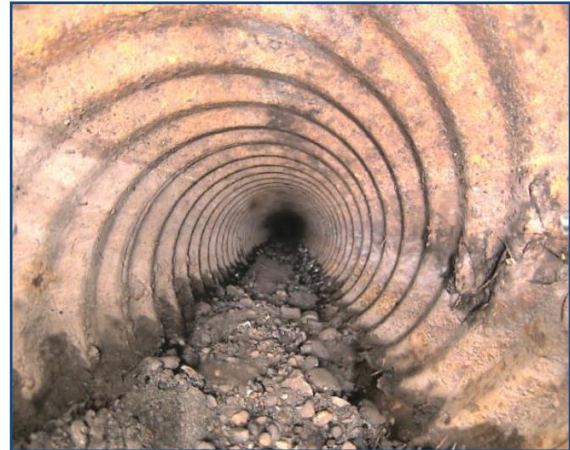
Debris in pipe invert (MOA ID 32996)
