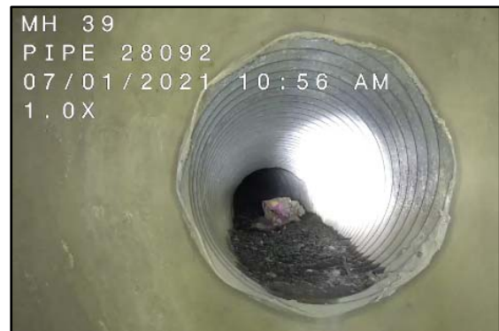
Photo 3 - Pipe 28092 (Sediment Buildup)
