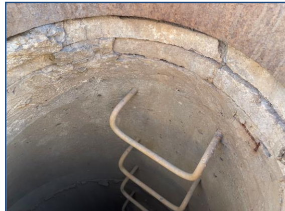
Cracked grade rings (MOA ID 1930-039)
