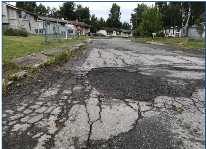
Curb heaving and significant pavement failure on 58 th Avenue
