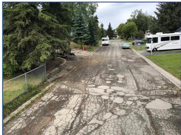
Poor roadway condition along 57 th Avenue
