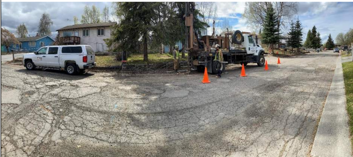
05/11/2021: Drill rig on BH-02 with utility markings prior to drilling. Borehole marked with white paint.
